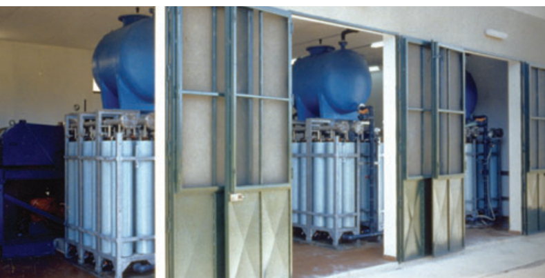
Sea water desalination system: 3 lines processing 500 m 3 per day.
